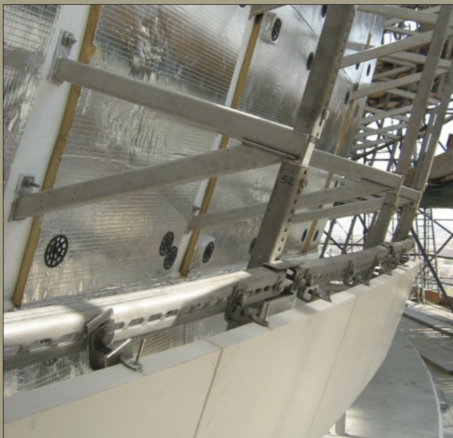
The sub channel system used for the installation of the domes, for which the stone had to be cut to curve in two radiuses with different radiuses on each course.
